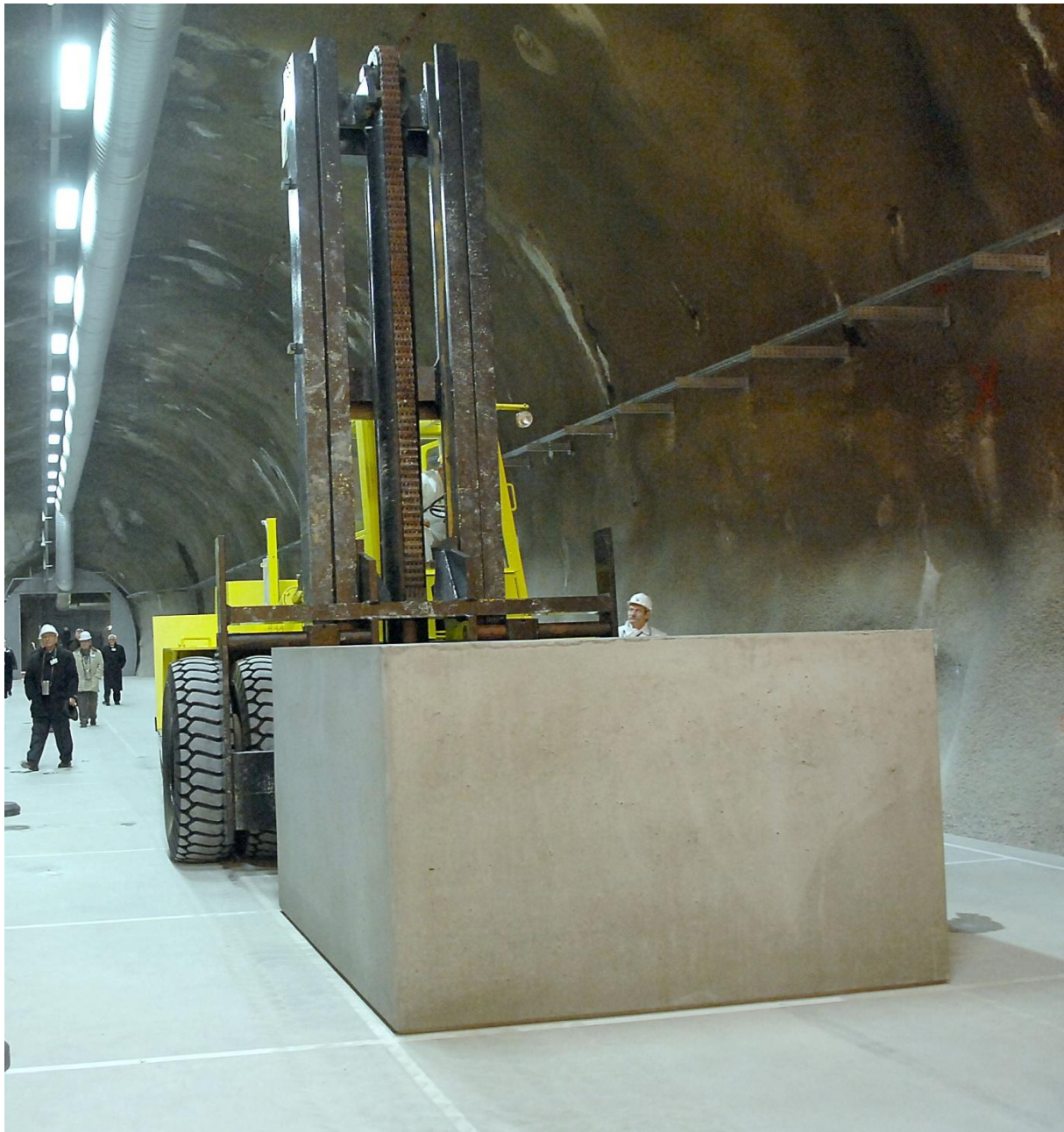
Figure H.3 – 2. Disposal of the first reinforced concrete container in the National Radioactive Waste Repository
