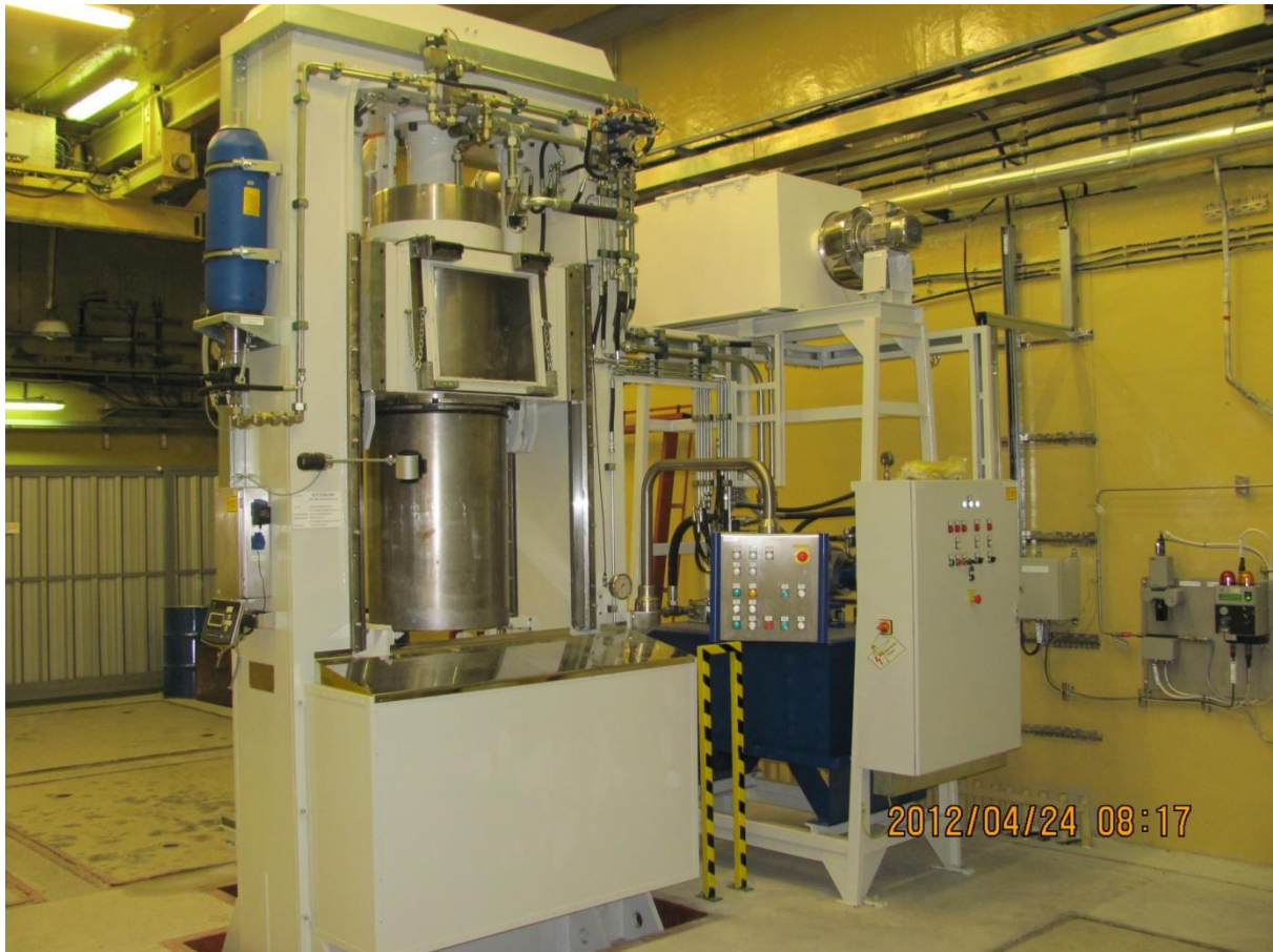
Figure D.2.4 – 2. Waste compressor machine
