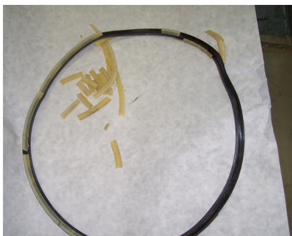
The worn out valve sealing
