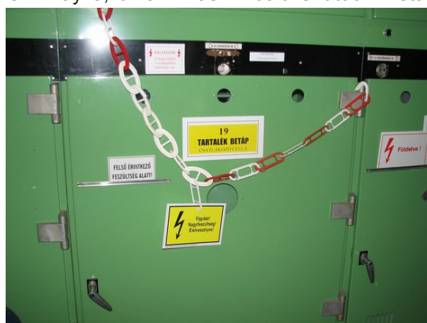
Indication of energized state of the cubicle №19
