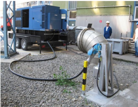
Mobile diesel generator (from Paks NPP education material)
