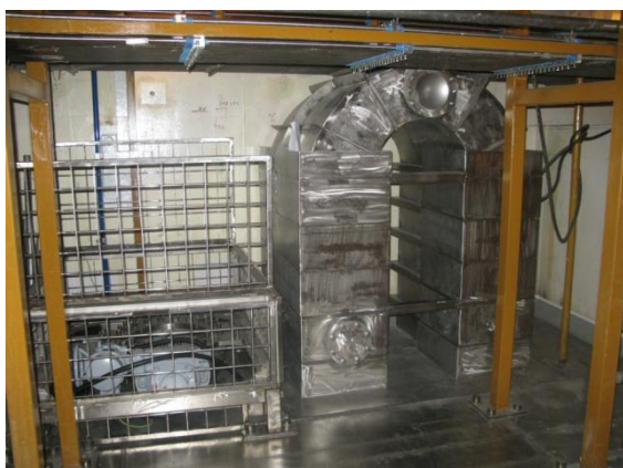
Water-lock (U-profile) of the ex-vessel cooling system. (from Paks NPP education material)
