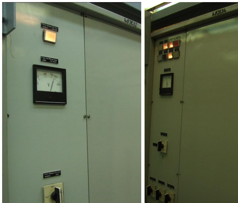
Switchboards affected by the event
