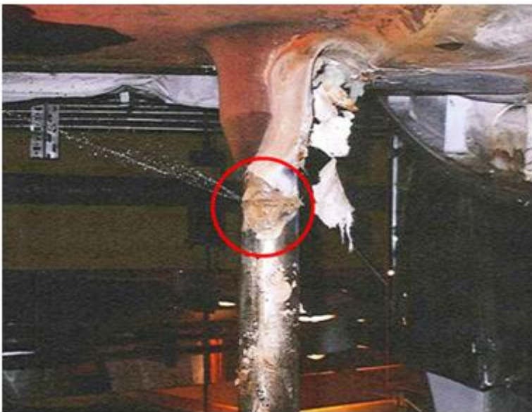
Leaking steam generator drainage nozzle with boric acid marks and some thermal insulation parts
