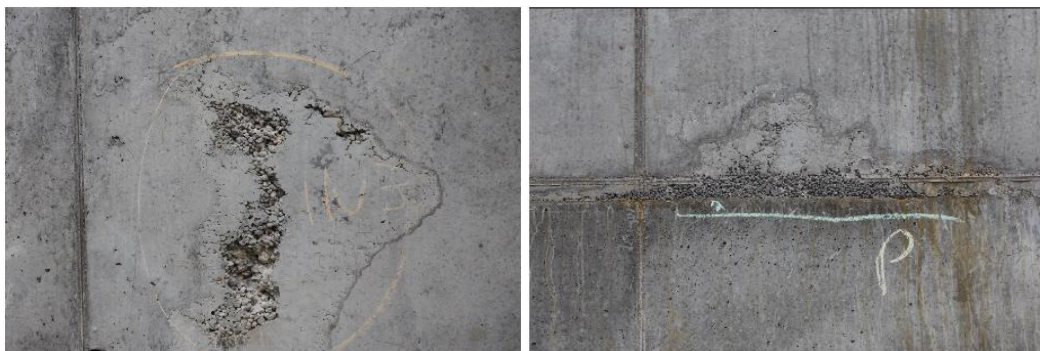
Concrete deficiencies in the ISFSF wall
